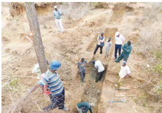
Community members participate in Laying out the foundation for construction of gabions
